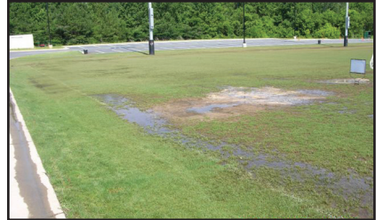
Poor field drainage on a soccer field improperly constructed. Photo: Tony L. Strickland, CSFM
