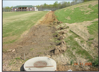
Example of bad conduit installation along edge of a natural turfgrass field and reconstruction to fix it. Photo: Tony L. Strickland, CSFM
